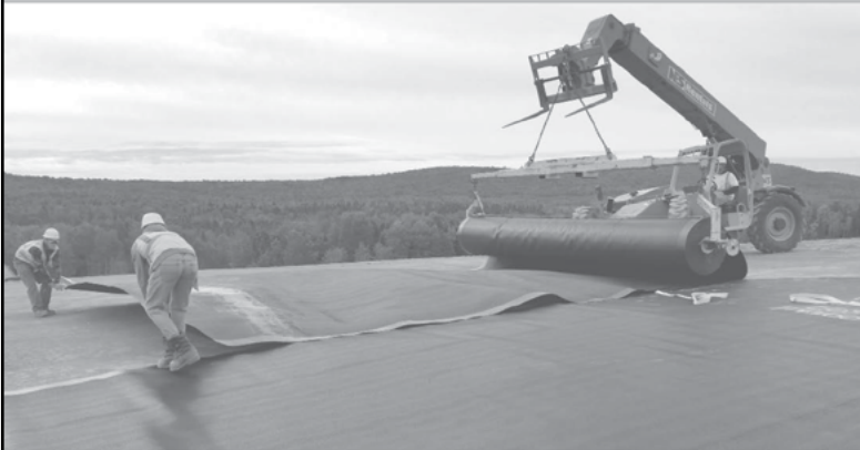
In 2015, the Presque Isle Landfill Closure project received an ACEC of Maine Engineering Excellence Award, a Governor’s Award for Environmental Excellence, and a Build Maine Award from AGC Maine.
